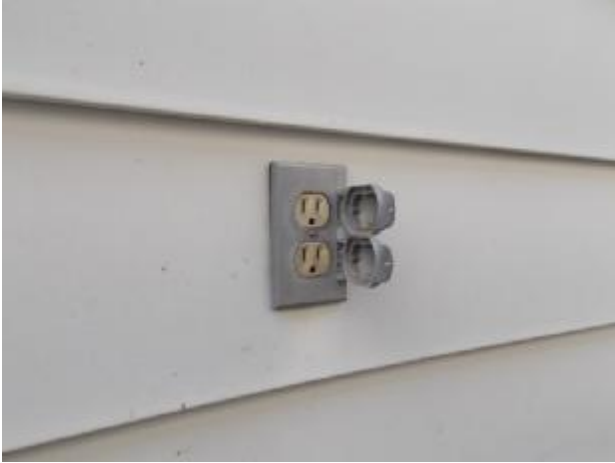
Defective outlet covers.
