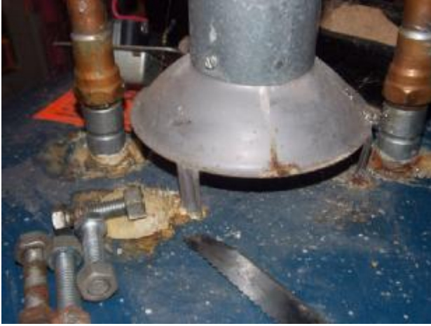
Rusted water heater.
