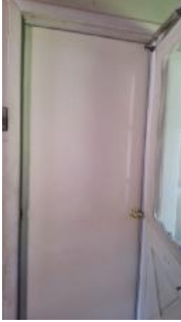
Improper fire door.
