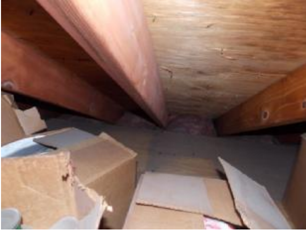
Insulation covering soffit vent.
