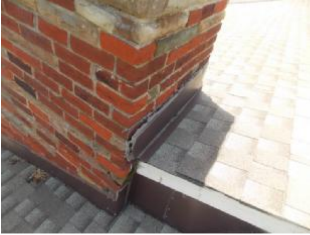
Failing chimney flashing.
