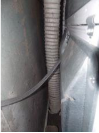
Torn vent tube.
