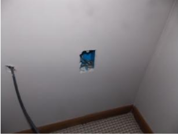
Exposed live electrical wire
